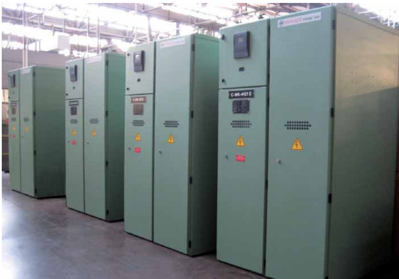
2 MVar - 12 kV - 50 Hz - PFC panels with switch and inrush current limiting reactors
