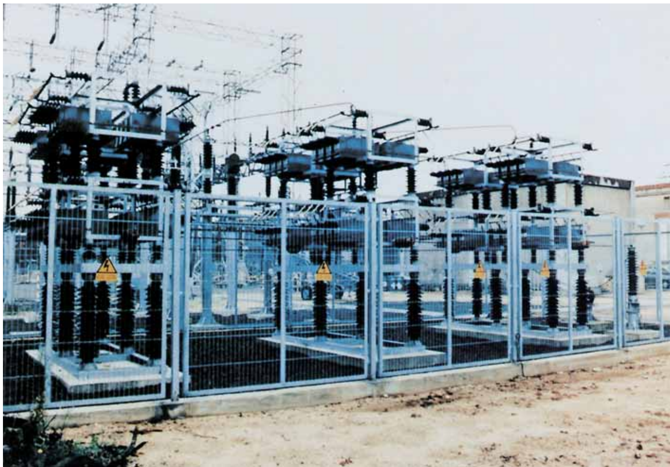
36 MVar - 110 kV - 50 Hz
